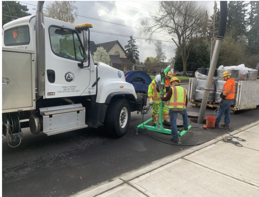
A Clark County Public Works crew replaces filter cartridges in an underground vault on Hazel Dell Avenue. Public Works' clean water division is proposing new stormwater rates to keep pace with required services. (Contributed by Clark County Public Works)
