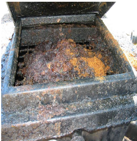
Grease trap in need of maintenance
