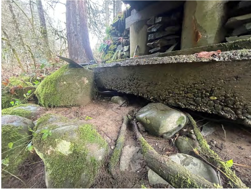
Photo 5 - Lewisville No 2 Rock filled spill through abutment with undermining.
