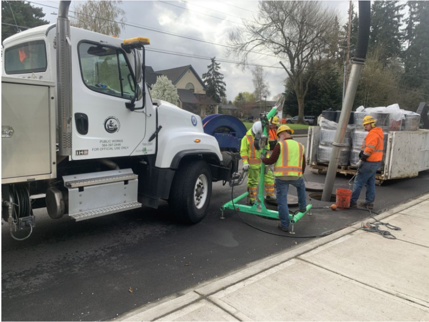
A Clark County Public Works crew replaces filter cartridges in an underground vault on Hazel Dell Avenue. Public Works' clean water division is proposing new stormwater rates to keep pace with required services. (Contributed by Clark County Public Works)
