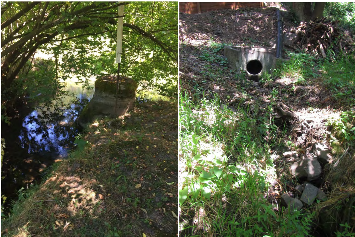
A manhole that is currently exposed in the main channel of Cougar Creek (left) and a stormwater runoff culvert lacking a rundown causing hillslope erosion (right) in Reach 12.
