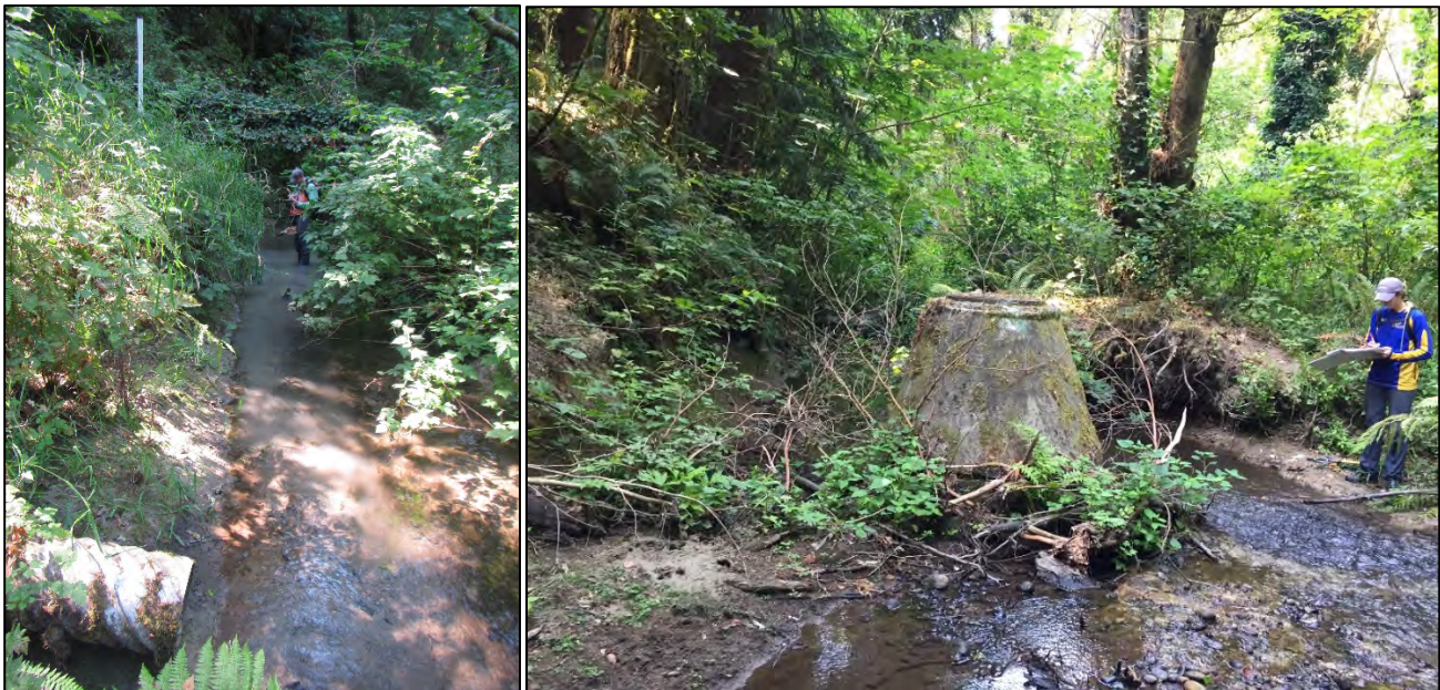
Exposed stormwater outlet within incised and straightened main channel (left) and an exposed manhole within the active channel of Cougar Creek (right) in the Cougar 3 project area.
