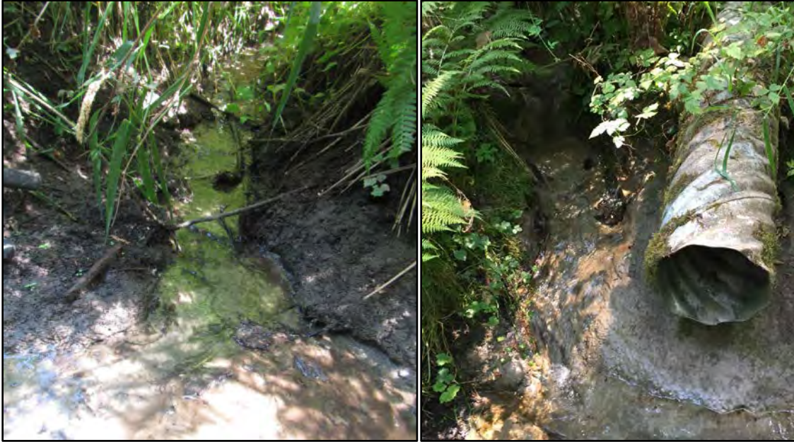
Figure 9. Examples of outfalls that lack energy dissipators and are eroding through the bank (left) and a gully that has formed adjacent to an outfall indicating that the outfall is not functioning.
