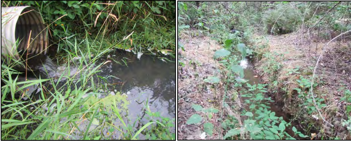
Figure 10: Perched culvert (left) and lack of channel complexity (right) limiting aquatic passage and habitat within the lower reaches of Suds Creek.
