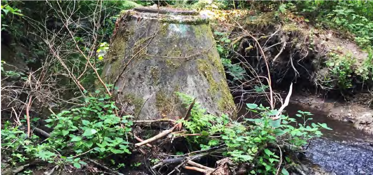
Figure 7: Channel avulsion and undercutting of existing waste water infrastructure along Cougar Creek.
