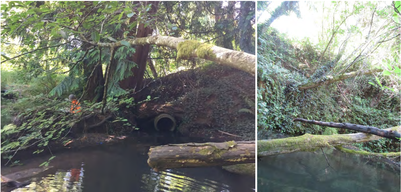
A flanked culvert (left) and significant bank erosion immediately downstream (right) in Cougar Creek in Reach 13.
