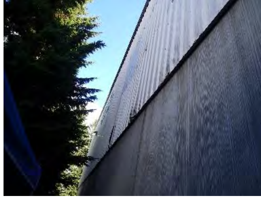
Figure 4 – Transfer Station, Damaged Metal Siding
