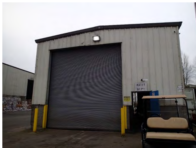
Figure 27: Damaged Siding Above the Rollup Door
