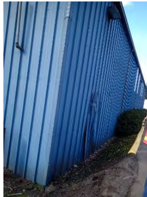
Figure 9 – Damaged Siding on HHW Building
