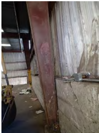
Figure 12 – Warped Steel Column Flanges
