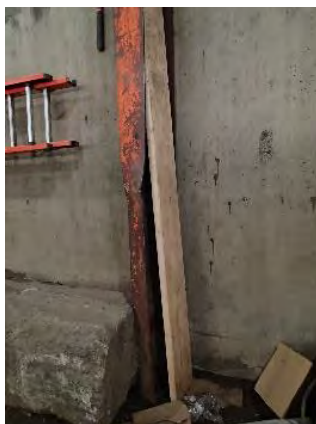
Figure 2– Warped Column Flange
