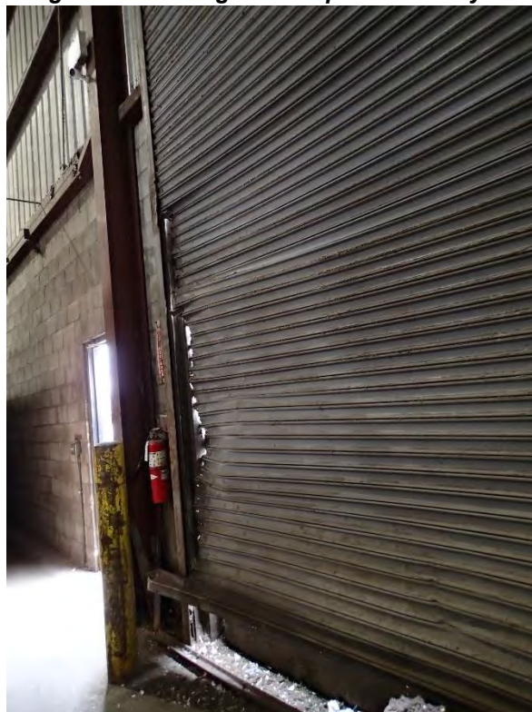
Figure 10: Damaged Rollup Door at Bay 12
