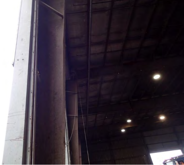
Figure 6: Damaged Column Flange at Commercial Unloading Bays
