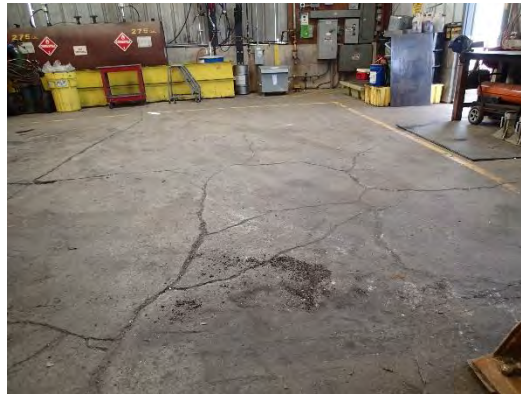
Figure 13 – Recycling Building’s Cracked Floor
