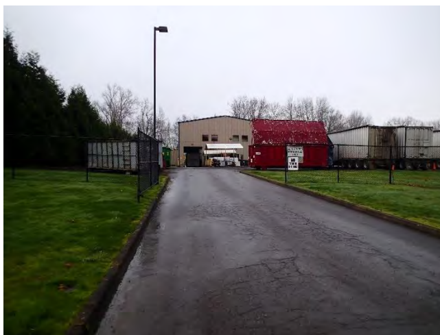
Figure 12: Cracked Pavement at Transfer Truck Exit
