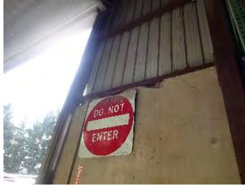
Figure 6 – Damaged Concrete Near Entrance
