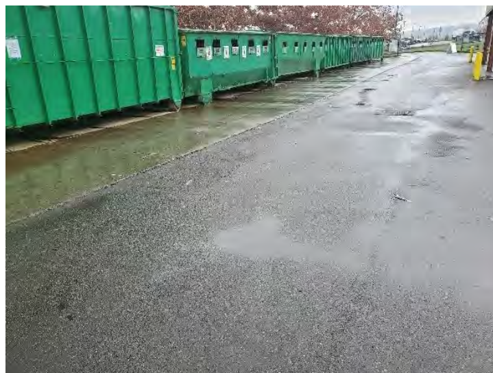
Figure 14: Cracked Pavement at Public Recycling Area
