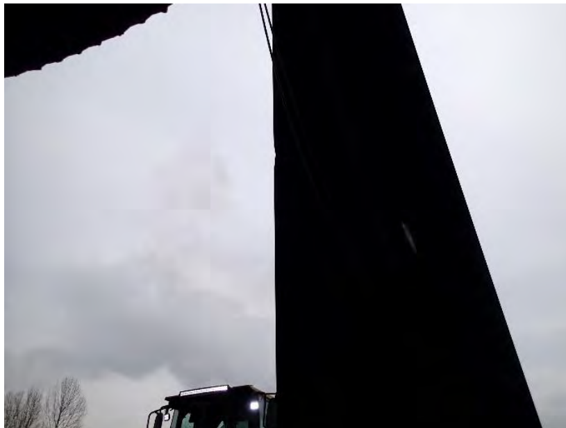
Figure 5: Damaged Column at Public Unloading Bays
