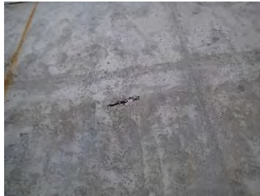
Figure 5 – Rust-Stained Exposed Reinforcements in Exterior Wall
