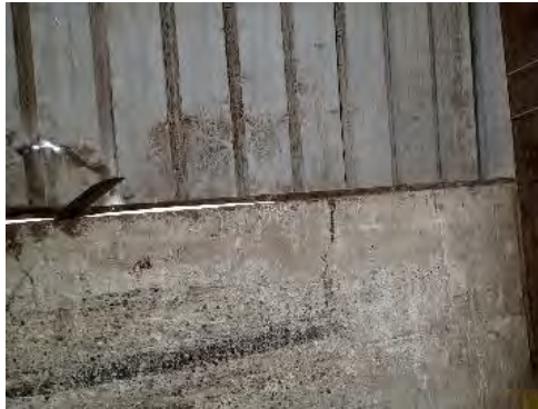
Figure 11– Cracked Concrete Wall
