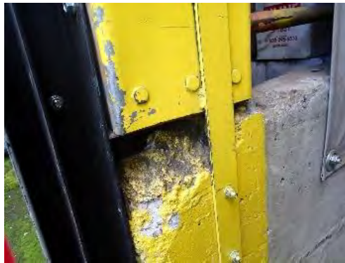
Figure 10 – Damaged Pier Supports on Recycling Building
