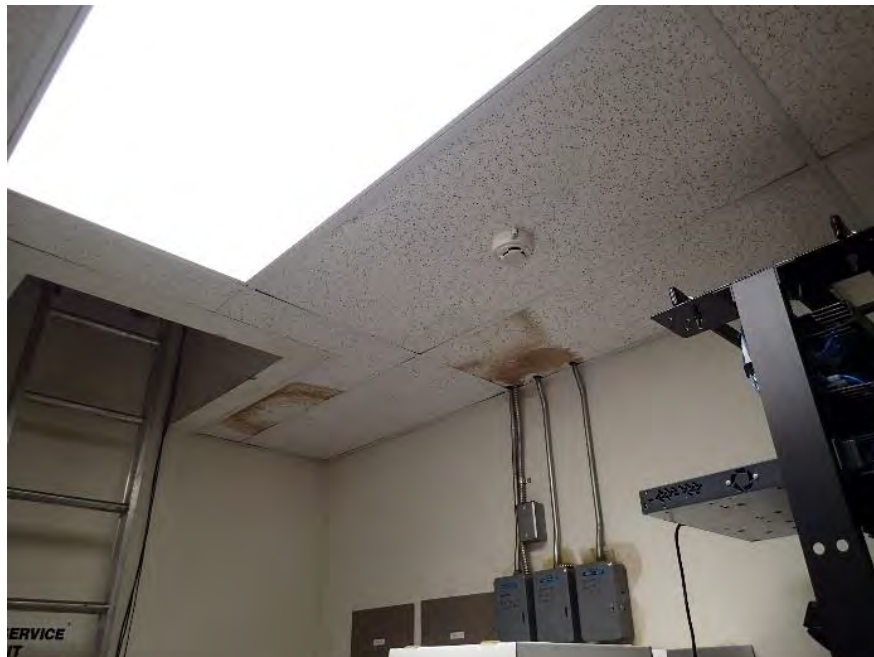
Figure 20: Water Stains on Ceiling Tiles
