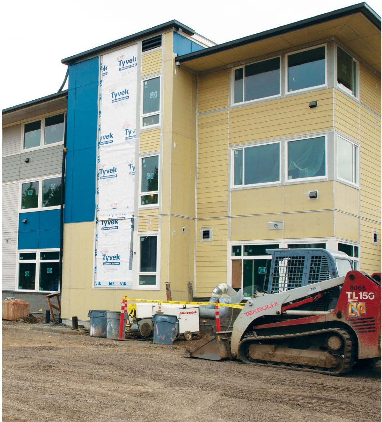
Construction of Meriwether Place with equipment in the foreground. Photo provided by Vancouver Housing Authority.
