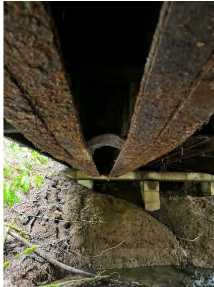
Photo shows significant rust on the steel girders as well as buckling of the plate between girders (looking south)
