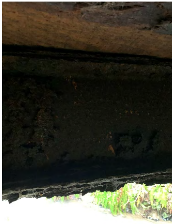
Photo shows significant rust on the steel girder (web and flanges)
