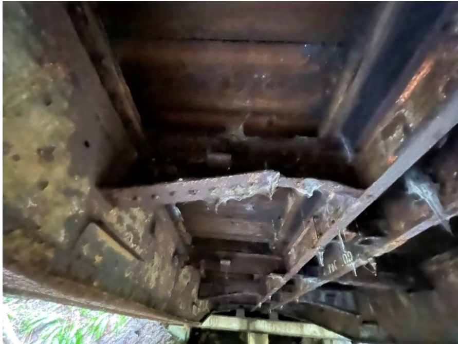
Photo shows significant rust on the steel connection elements, girders and steel diaphragms
