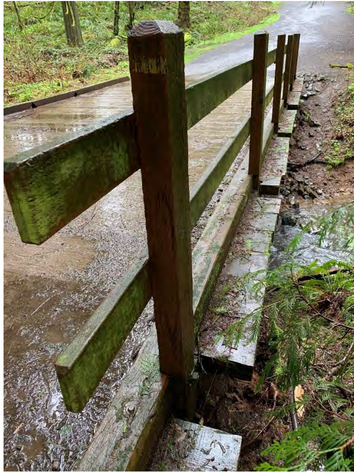
Photo shows deterioration of the timber deck as well water ponding on the deck
