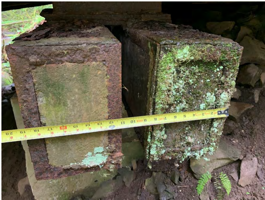
Photo shows vegetation and moss growth on pier cap beams
