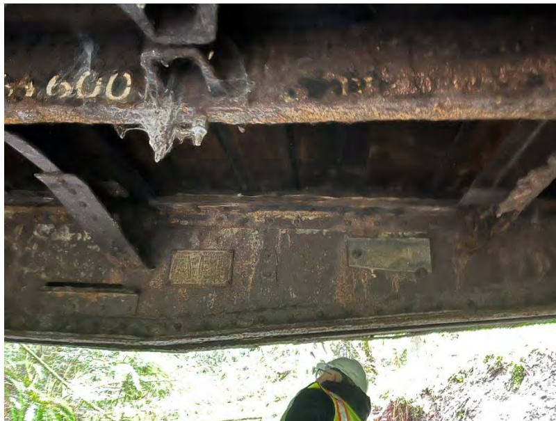
Photo shows significant rust on the steel girders
