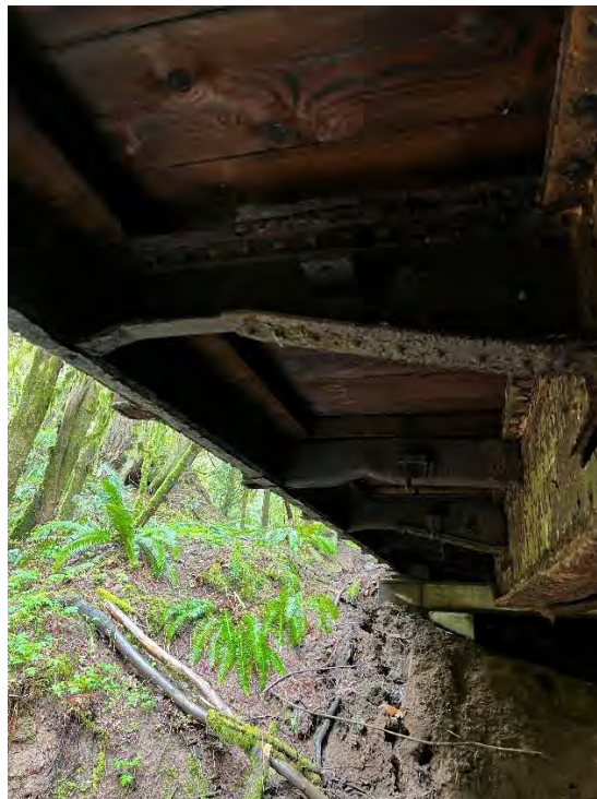
Photo shows significant rust on the steel girders as well as steel diaphragms
