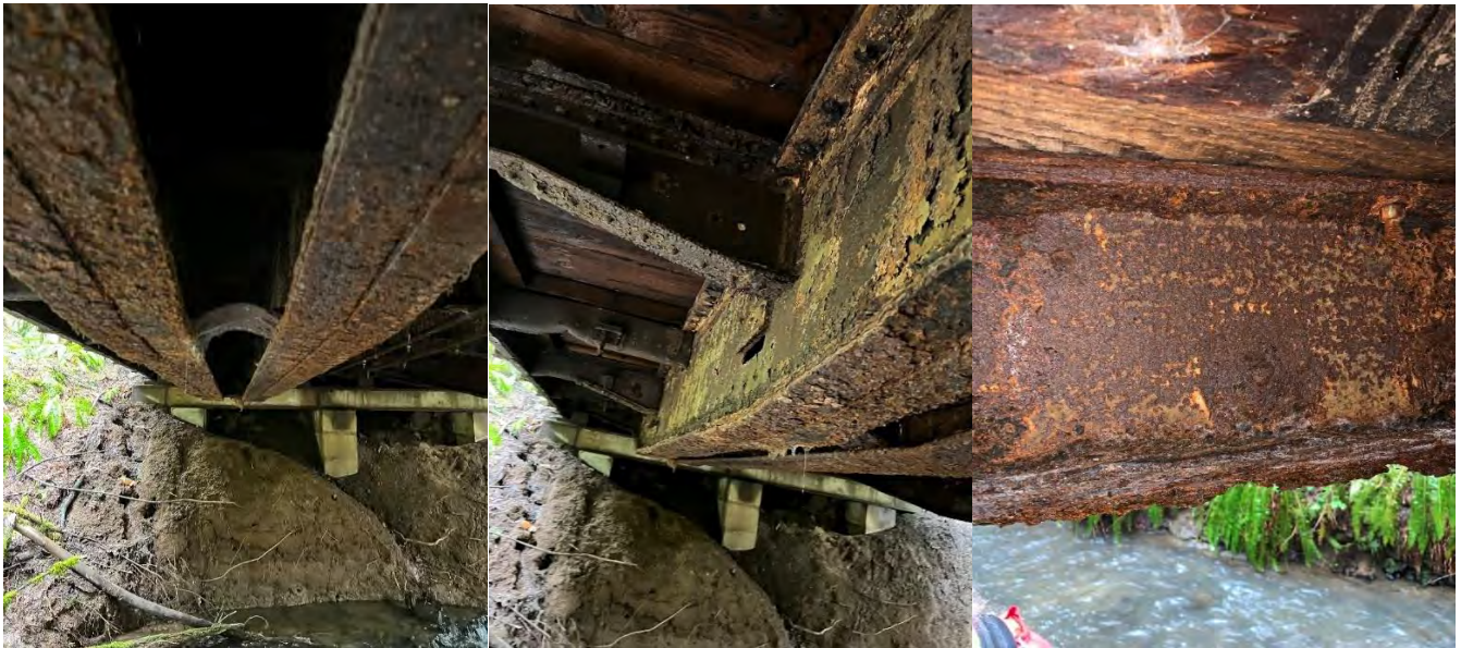
Representative photos illustrating significant rust on the steel girders, diaphragms, connection elements, and buckling of the plate between girders
