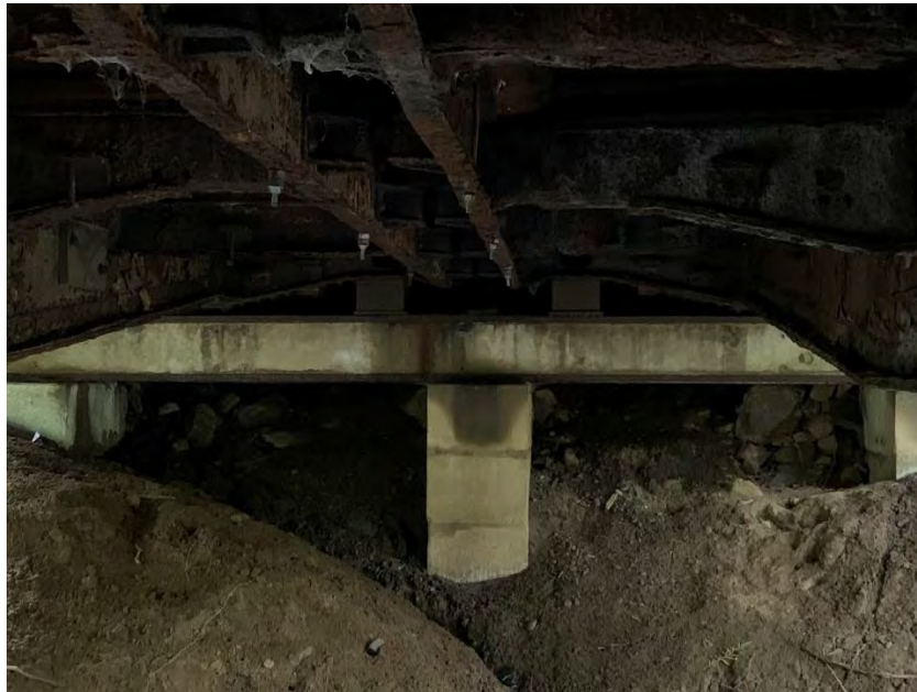
Photo shows significant rust on the steel connection elements, girders and steel diaphragms
