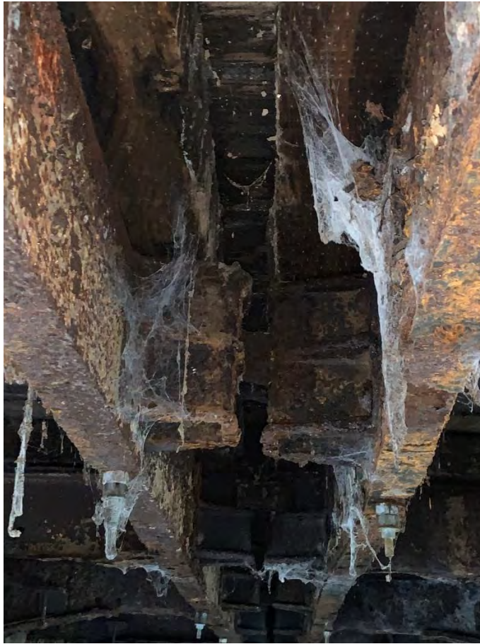
Photo shows significant rust on the steel connection elements, girders, and steel diaphragms
