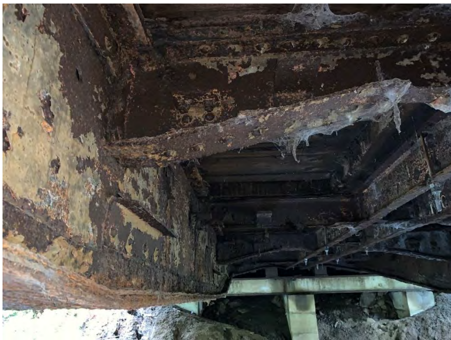
Photo shows significant rust on the steel connection elements, girders, and steel diaphragms
