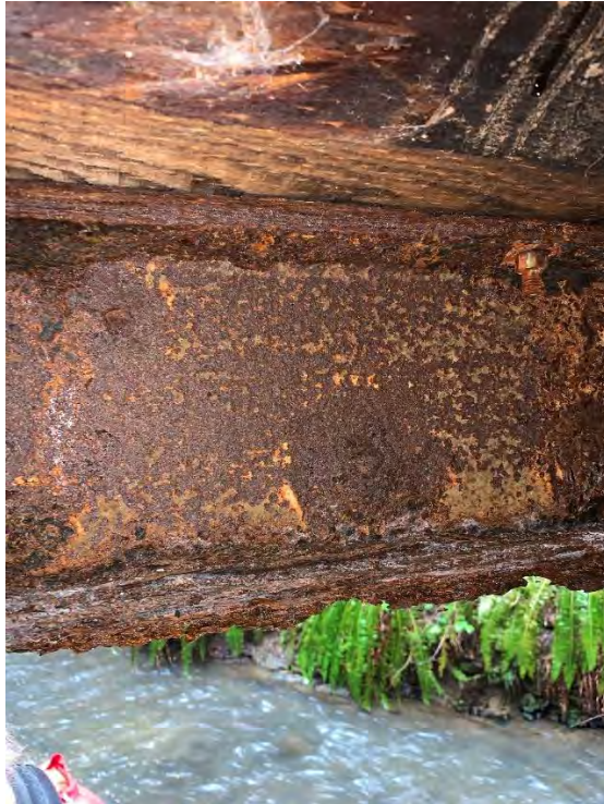
Photo shows significant rust on the steel girder (web and flanges)
