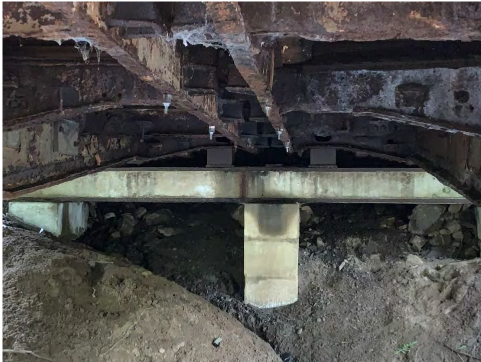
Photo shows significant rust on the steel connection elements, girders and steel diaphragms
