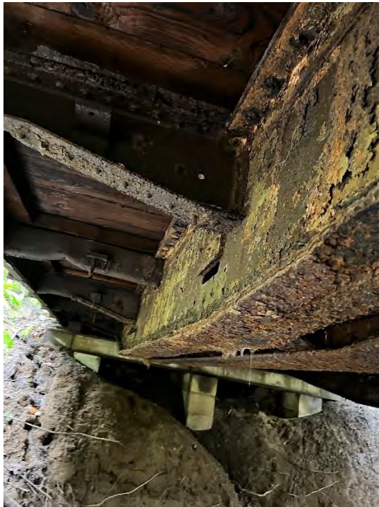
Photo shows significant rust on the steel connection elements, girders as well as steel diaphragms
