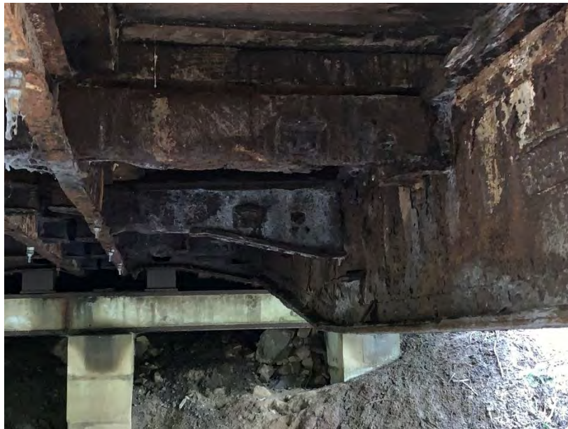
Photo shows significant rust on the steel connection elements, girders and steel diaphragms
