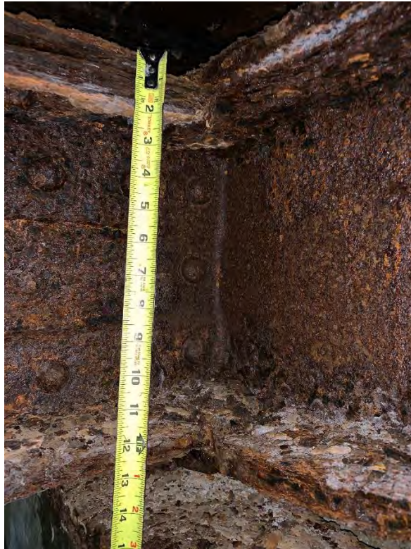
Photo shows significant rust on the steel connection elements
