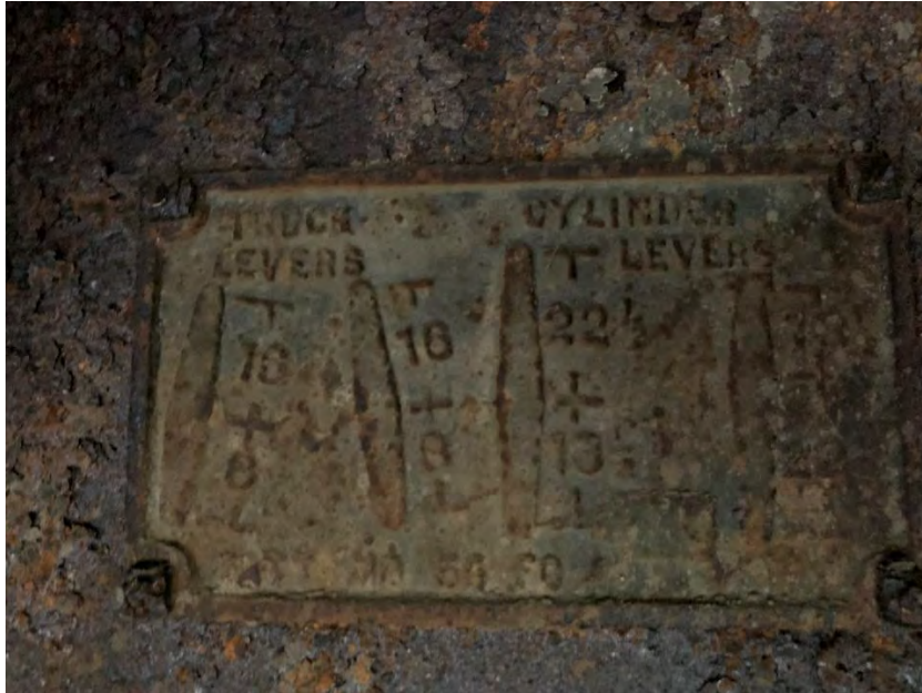
Photo shows significant rust on the steel element
