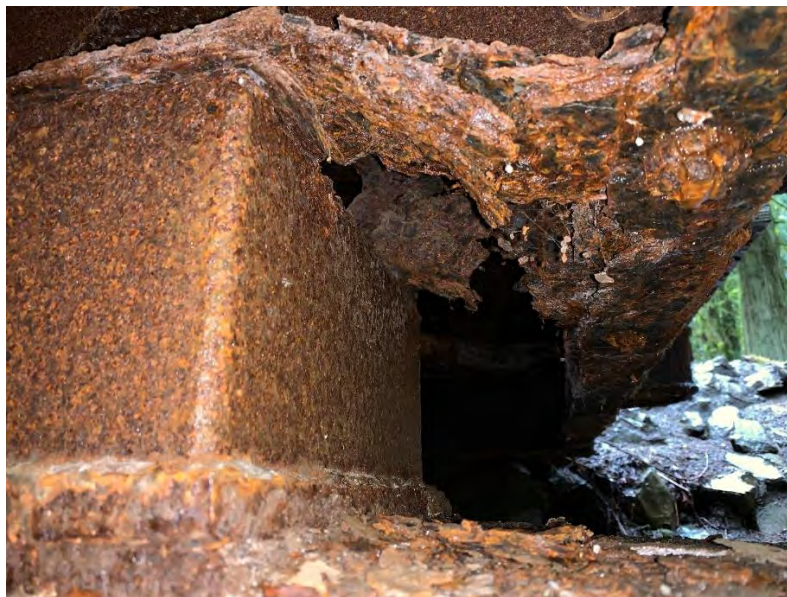
Photo taken at the abutment shows significant rust on the steel connection elements, steel diaphragms and diaphragm support blocks over pier cap
