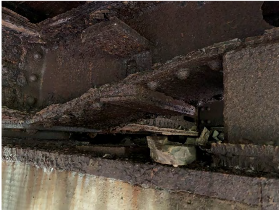
Photo taken at the abutment shows significant rust on the steel connection elements, girders, diaphragm support blocks, and steel diaphragms
