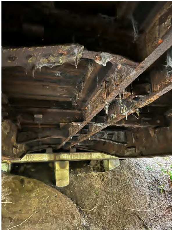
Photo shows significant rust on the steel connection elements, girders as well as steel diaphragms
