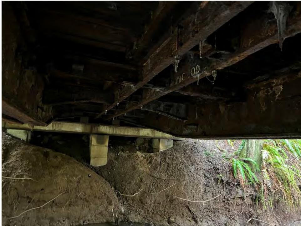
Photo shows significant rust on the steel connection elements, girders as well as steel diaphragms
