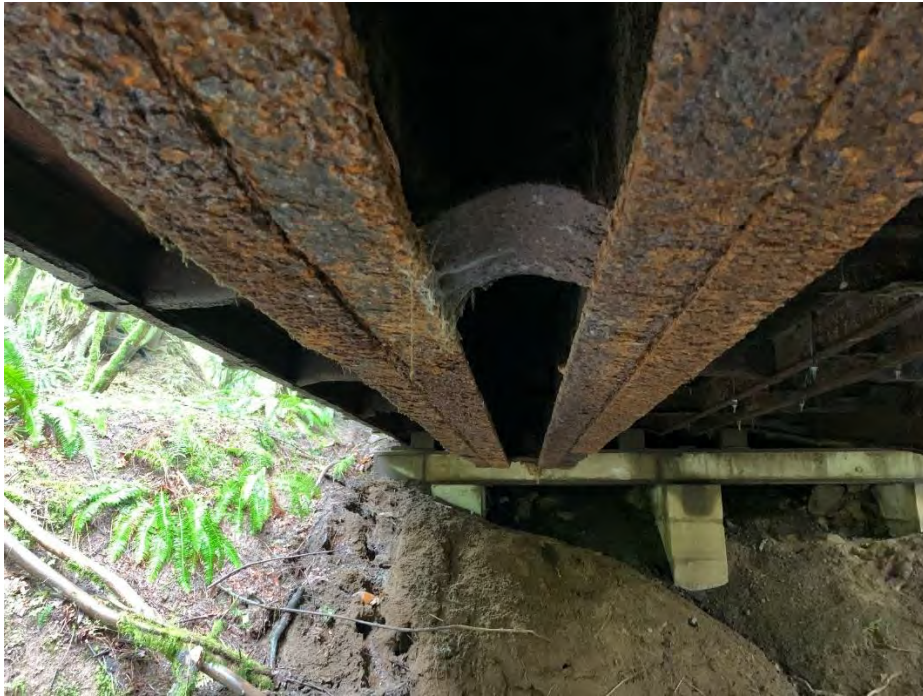
Photo shows buckling of the plate between girders, significant rust on the steel connection elements, girders, and as steel diaphragms
