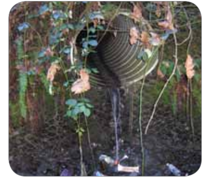
Untreated runoff and trash
