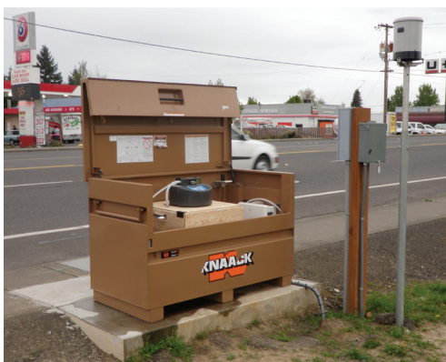
Stormwater monitoring equipment
