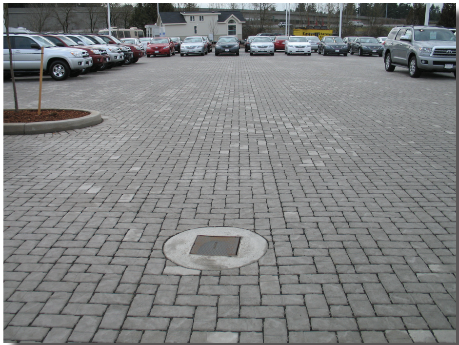
Monitoring well in permeable pavement
